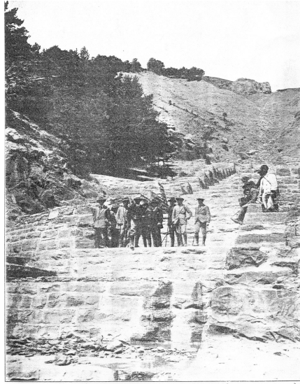
Figure 4. On the left branch a channel of 179 m length was built, with 32 steps, and variable width.
